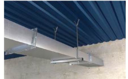
Ventilation duct on trapezoidal sheet
