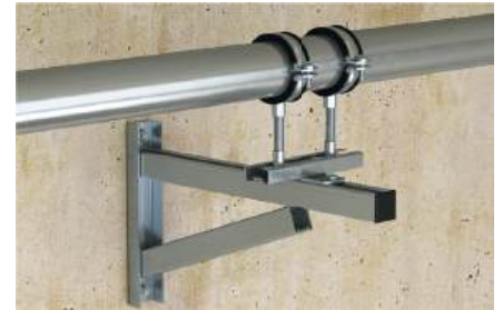
Media lines with thermal expansion
