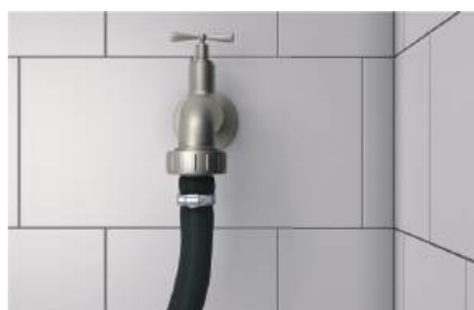
Outlet valve with hose
