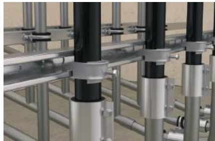
Supply lines fixed to FUS channel
