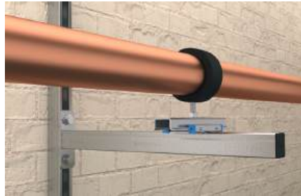
Refrigerant pipe clamp on sliding element
