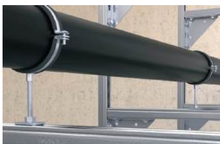
Connection on channel
