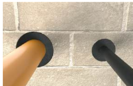
Insulated and combustible pipes
