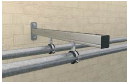
Pipelines on cantilevers
