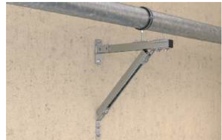
Upright pipe on cantilever arm
