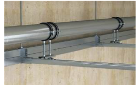
Media lines with thermal expansion
