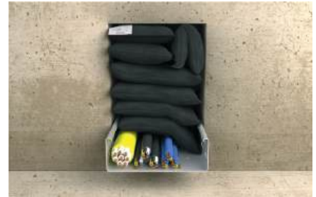
Electrical wall application
