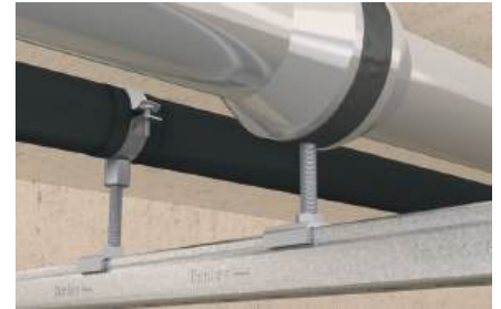
Refrigerant pipe clamps
