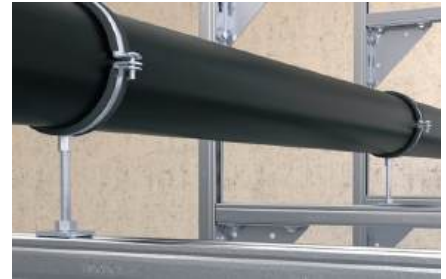
Connection on channel
