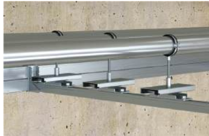
Media lines with thermal expansion
