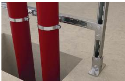
Waste water pipe
