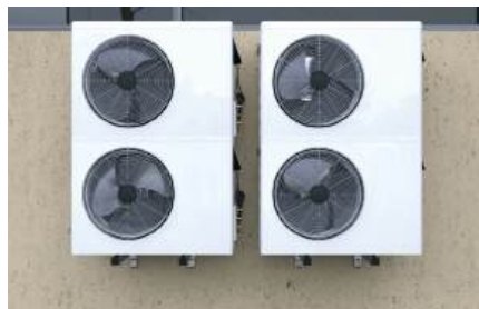
Air conditioning units
