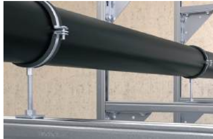
Connection on channel
