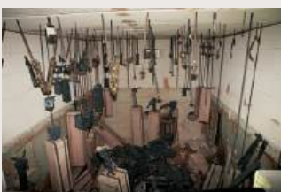
Fire inspection after.
