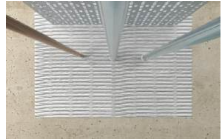
Mixed penetration through the wall
