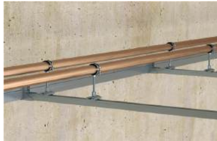
Media lines with thermal expansion
