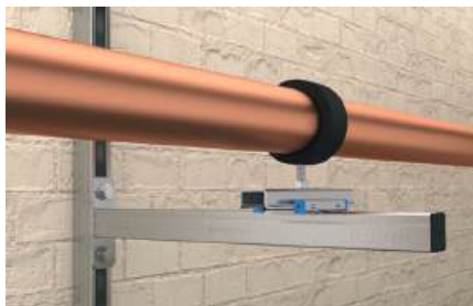
Refrigerant pipe clamp on sliding element
