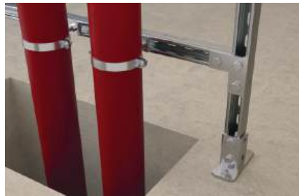
Waste water pipe
