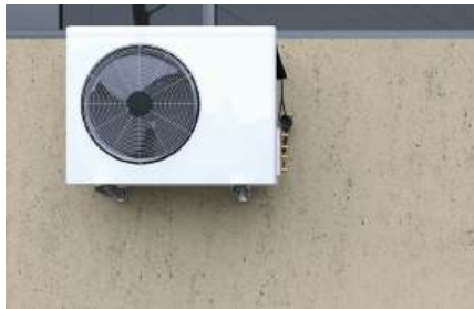
Air conditioner on the outer wall
